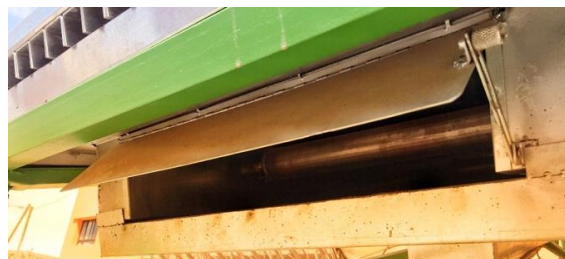
Figure 8. Air vent for gas combustion.
